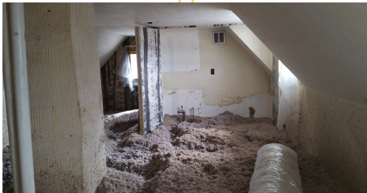
Engineers evaluated the Library for safety and load-bearing. They declared that the second story, "Shall not be occupied or used for storage." Therefore, it is an unoccupied attic space; insulation was blown in to save on energy costs.
