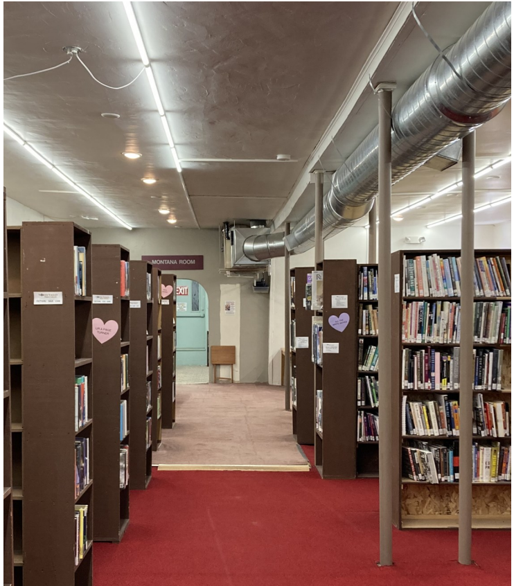
This photo illustrates the lights in the back going out because of the movement in the ceiling, the uneven floor, and the poles, from the cellar to the ceiling, that keep up the second floor up.
