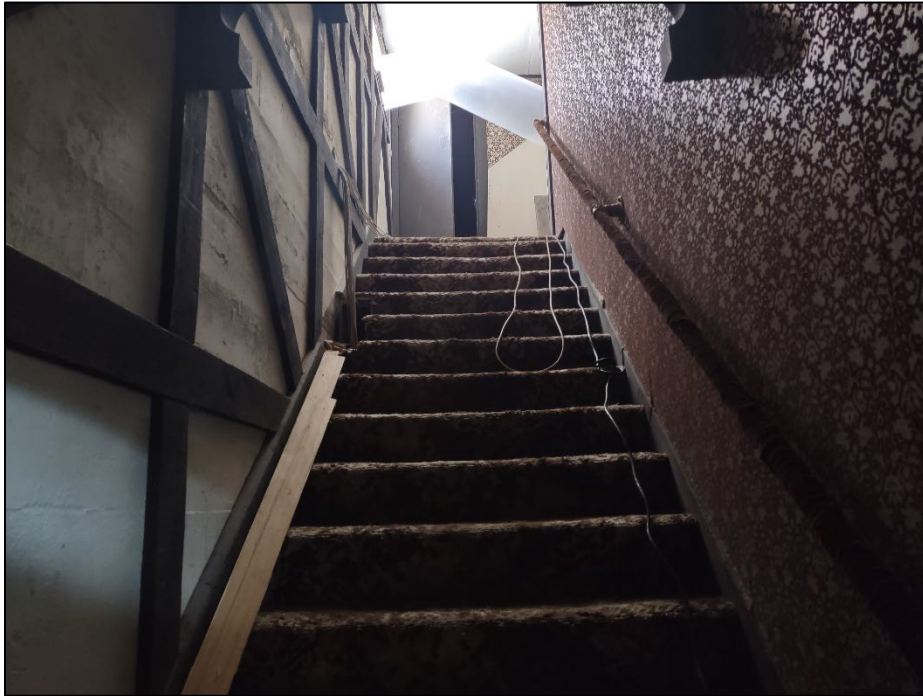
Photo 9. July 29, 2024. Upper Floor Roofing Spill. Containment was installed at the entrance to the storage room at the top of the stairwell. On the floor of the storage room is asphalt roofing mixed in with paper insulation. Negative air was installed with venting out of a HEPA filter discharged out a second story window.
