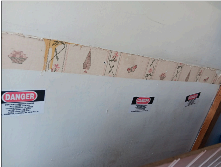
Photo 6. July 29, 2024. Wallpaper Main Level: Warning signage attached to plaster near the wallpaper containing ACM.
