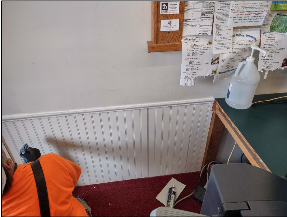
Photo 7. July 29, 2024. Wallpaper Encapsulation. Wood paneling covering the wallpaper and danger signage. The paneling edges were siliconed to prevent air gaps in the encapsulation. The paneling should be inspected six months after encapsulation and every year after.
