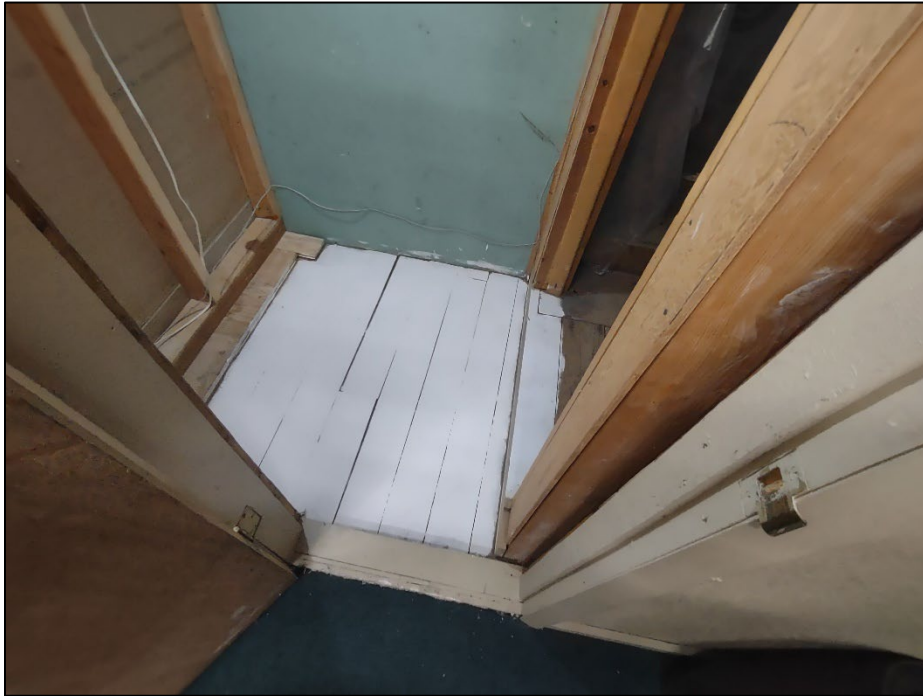
Photo 5. July 29, 2024. LBP Wooden Floor: The LBP covered floor was scraped and vacuumed to remove paint and debris before three coats of Fiberlock LBC were applied to encapsulate the LBP. The paint should be inspected six months after encapsulation and every year after.
