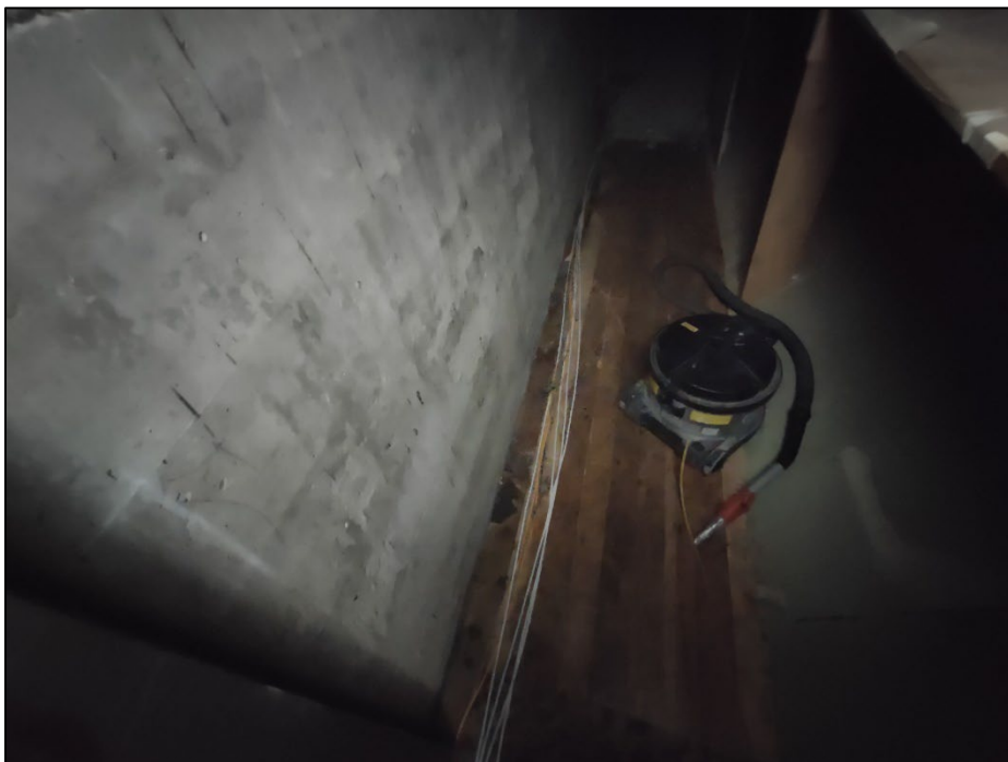
Photo 10. July 29, 2024. Upper Floor Roofing Spill. The storage room floor and surfaces were vacuumed (with HEPA filter) and wet wiped to remove the asphalt roofing material.
