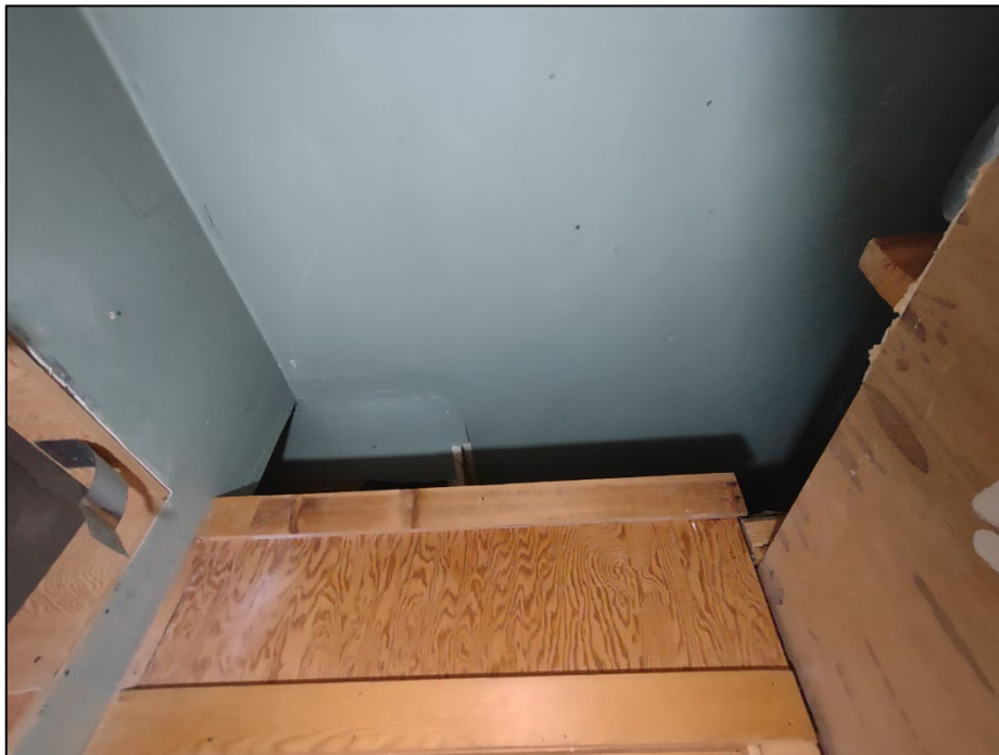
Photo 4. July 29, 2024. Damaged drywall ceiling: post cleanup of the spilled damaged ceiling drywall. The area was vacuumed (with HEPA filter) and wet wiped.
